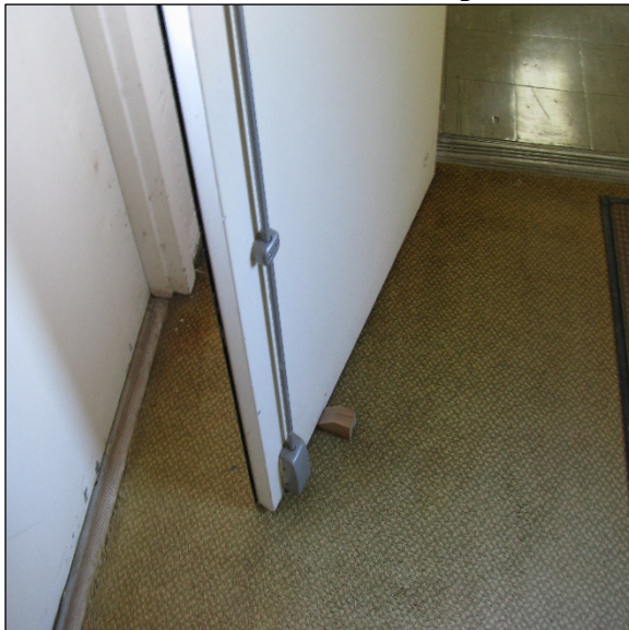
Fire Door Shimmed Open
