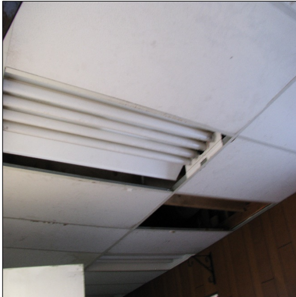
Missing Ceiling Tiles and Light Diffuser
