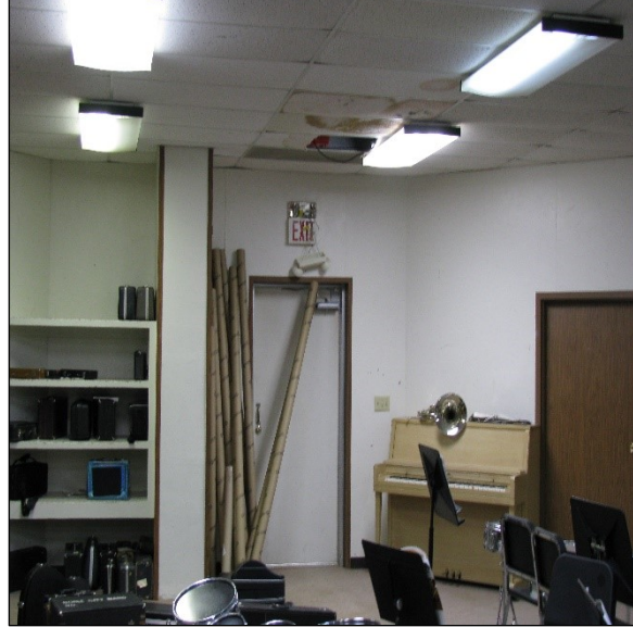
Fire Door Blocked and Broken Exit Sign
