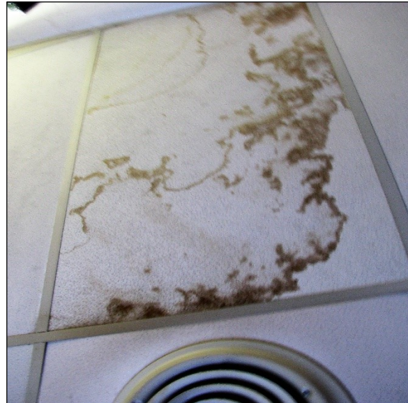
Stained Ceiling Tile Typical
