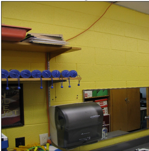
Extension Cords Used as Permanent Wiring
