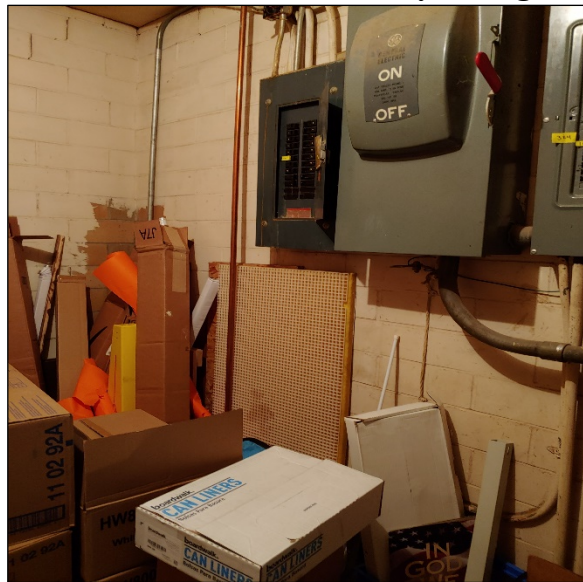
Electrical Panels blocked by Storage
