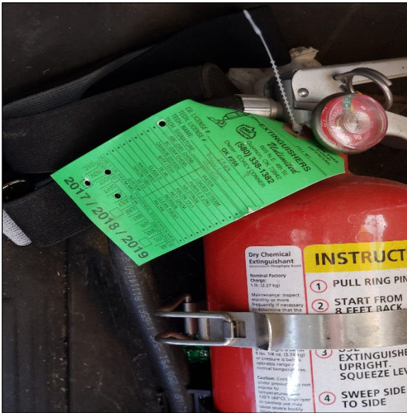
Out of Date Inspection-Fire Extinguisher
