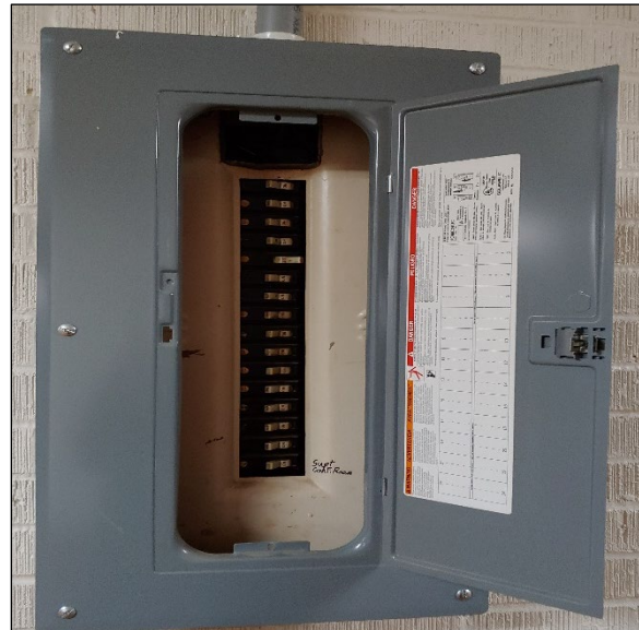
Altered Electrical Panel
