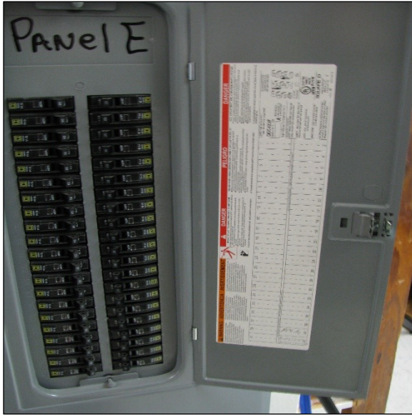
Unmarked Electrical Circuits in Panel
