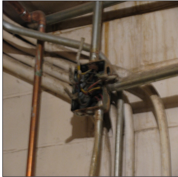
Open Electrical Junction Box
